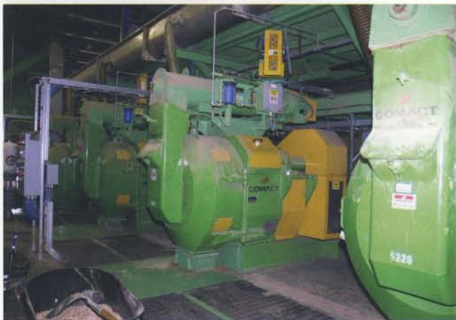
Pelletizing is via five Promill pellet mills supplied by Comact. The mills are designed for fast maintenance access and to avoid lubricant contamination of the final product.
